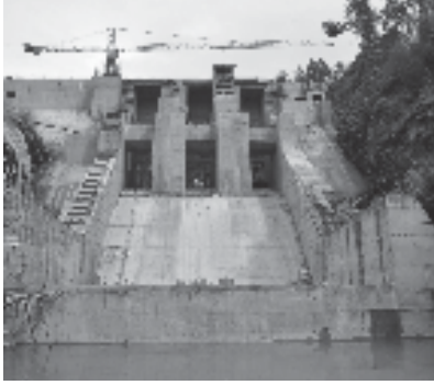
Parbati HE Project, Stage-II 83.7 m high Concrete Gravity Dam at elevation 2200 m
